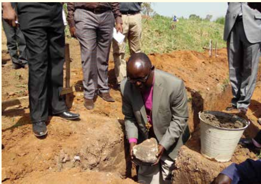
Archbishop (Rtd) Isingoma (DRC) lays the puts first stone of the Business Center for Agape, which is being set up as a Youth Empowerment Centre.
